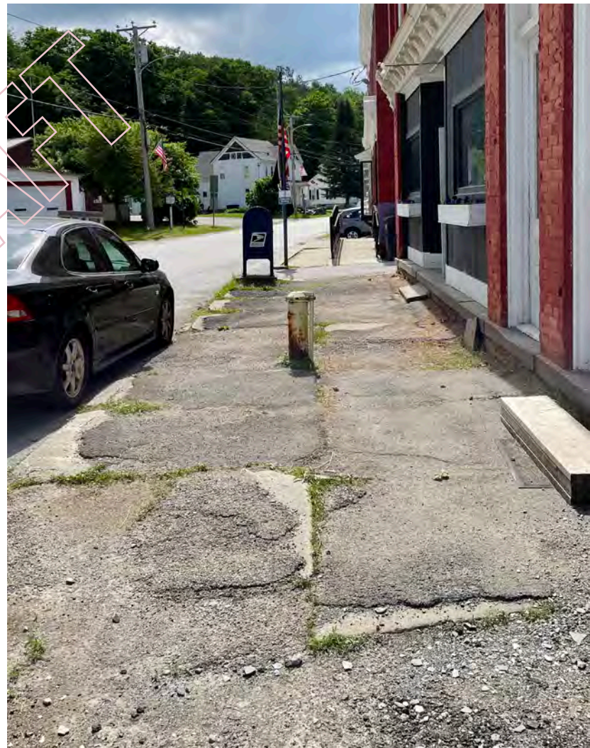
▲ Existing Sidewalks. The existing sidewalks in front of the Celery Compound (former Fish & Game building) and Post Office are in an advanced state of disrepair. The water wellhead which serves the Celery Building can be seen protruding up in the middle of the sidewalk, creating a potential hazard.
