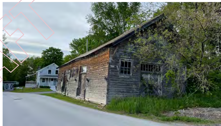
▲ Railway Shed. Railway freight shed, contributing historic structure circa 1890 featuring original stickwork and extended rafter tails. Unfortunately, due to the building’s proximity to the road, the rafter tails and corresponding roof overhang were cut off to avoid vehicle collisions. Currently vacant, ownership in dispute.
