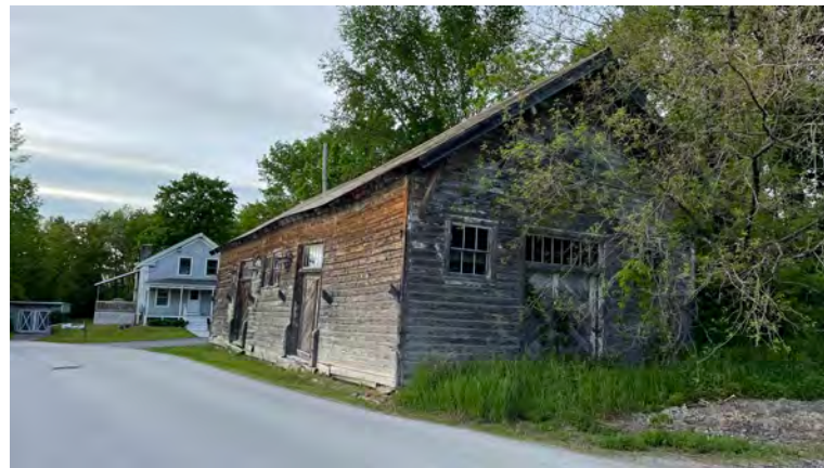
▲ Railway Shed. Railway freight shed, contributing historic structure circa 1890 featuring original stickwork and extended rafter tails. Unfortunately, due to the building’s proximity to the road, the rafter tails and corresponding roof overhang were cut off to avoid vehicle collisions. Currently vacant, ownership in dispute.
