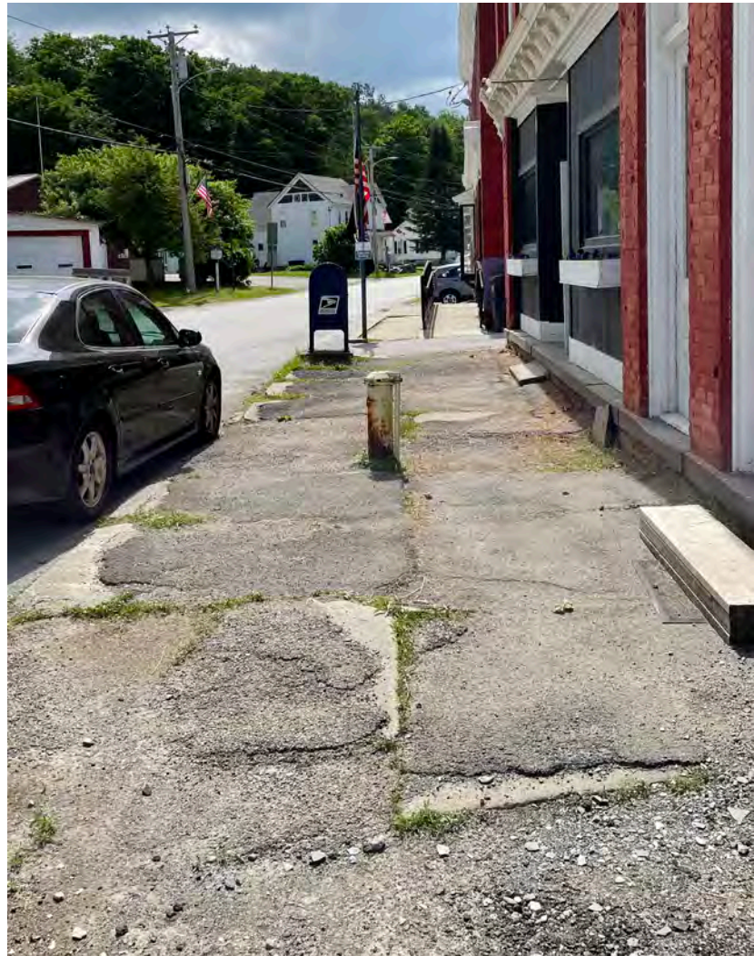
▲ Existing Sidewalks. The existing sidewalks in front of the Celery Compound (former Fish & Game building) and Post Office are in an advanced state of disrepair. The water wellhead which serves the Celery Building can be seen protruding up in the middle of the sidewalk, creating a potential hazard.
